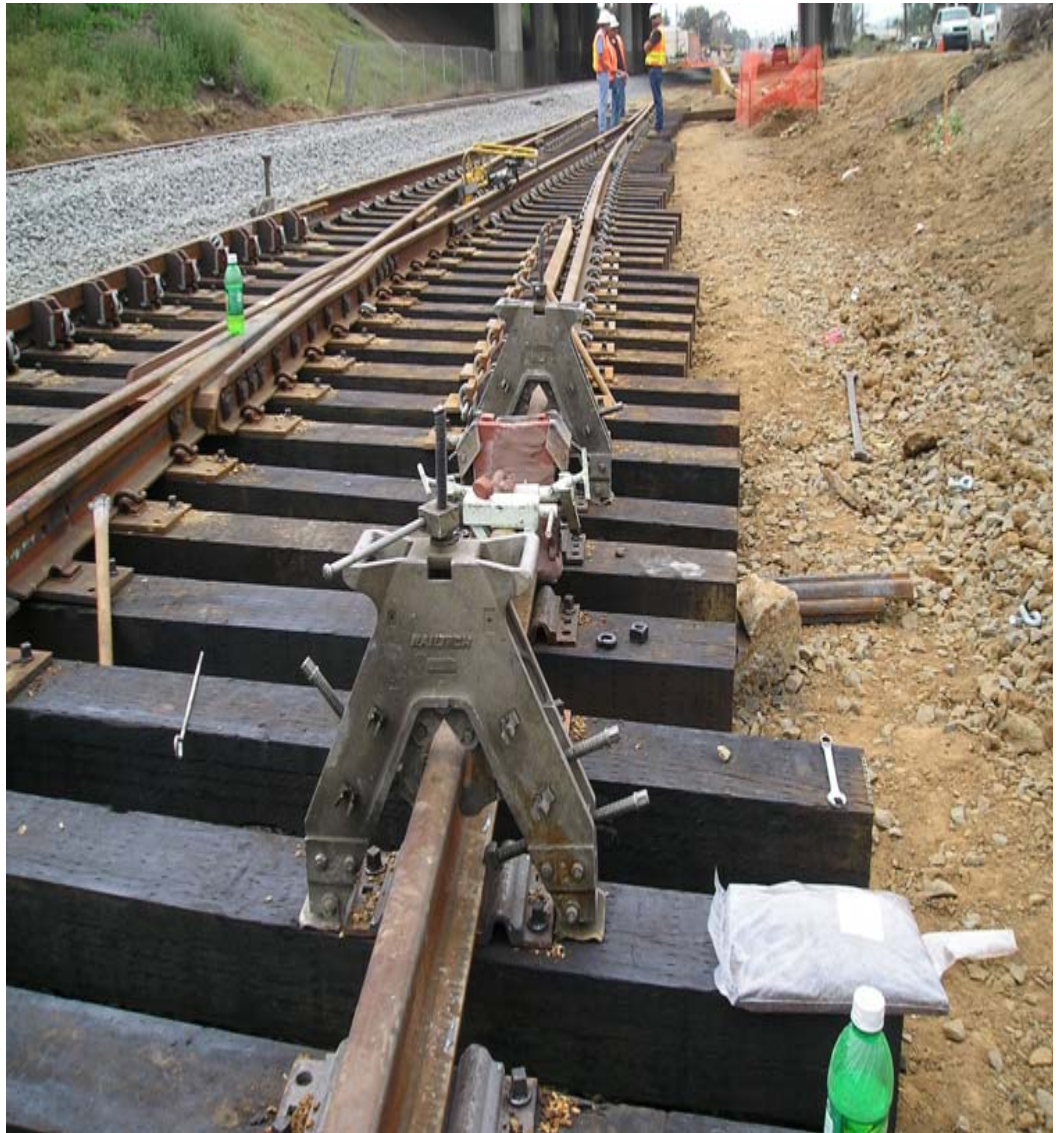
Left Handed Turnout
